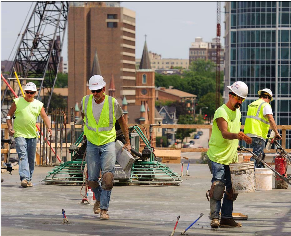
Pension capital invested by the HIT is keeping union construction workers busy from coast to coast. Shown here are workers at Milwaukee's $56.7 million Moderne development, one of 23 projects currently under construction or preparing to start up with HIT financing.
