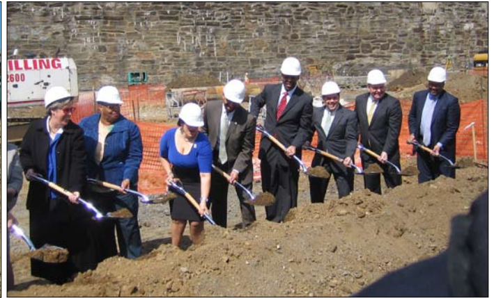
Paseo Verde, Philadelphia: Philadelphia Mayor Michael A. Nutter was joined by city, business, and community representatives for the groundbreaking at the project site adjacent to the Temple University Train Station.
