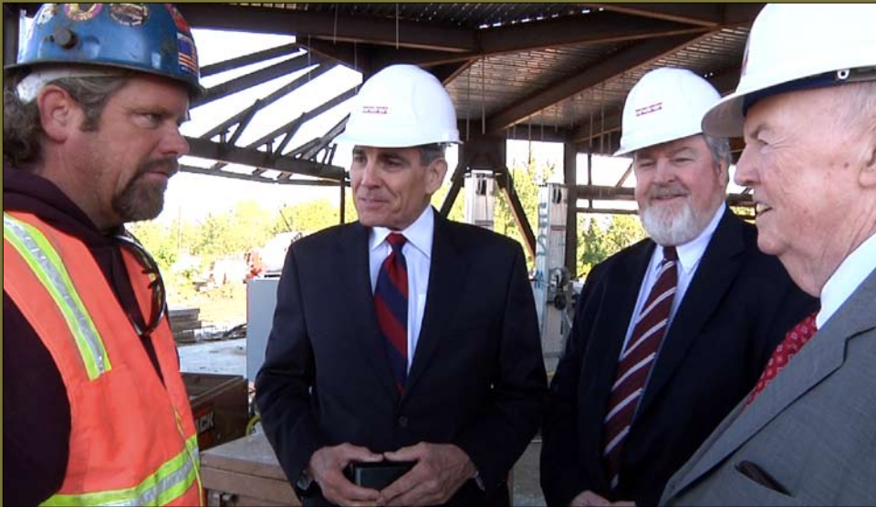
AFL-CIO President Emeritus and HIT Chairman John Sweeney (at right) talks with Daniel Quinn (left), Metallic Lathers Local 46, at the construction site of the HIT-financed Elizabeth Seton Pediatric Center in Yonkers, NY. Also touring the site are Paul Ryan (2nd from right), President of the Westchester and Putnam Counties Central Labor Body, AFL-CIO, and HIT's representative Mike Arnold. The project is generating approximately 800 union construction jobs. (more on page 2)
