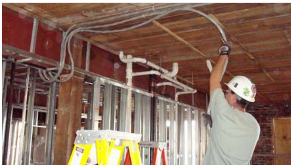
New electric power lines are run to units at the Hadley Apartments during the $15.8 million renovation of a former furniture store in Worcester, Massachusetts. The recently completed HIT-financed project generated approximately 100 union construction jobs.
