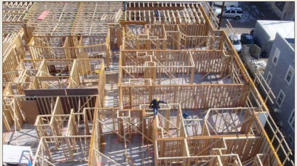
The HIT is creating employment for members of the local building and construction trades in the Minneapolis/St. Paul area with $25.9 million in financing for the 60-unit Solhem Apartments (above) and the 103-unit Inver Glen Senior Housing development. The estimated 200 jobs represented by these projects bring the total number of union construction jobs created by HIT investments in Minnesota to over 5,000.
