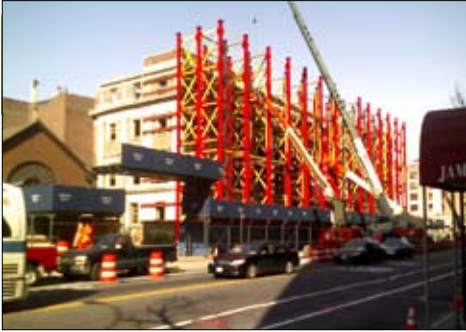
Construction is underway at the $165 million Queens Family Courthouse mixed-use development in Queens, NY, part of the HIT's New York City initiative. The project is generating over 1,000 jobs for members of the local building and construction trades.
